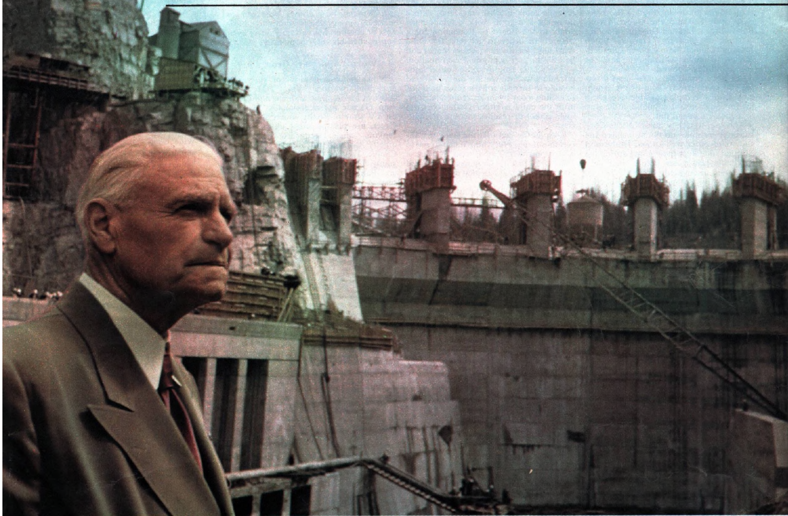
Morrison at the Cabinet Gorge power installation in Idaho. Before building the dam, he handled perhaps the toughest river conversion job
